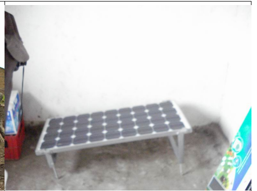
Solar Panel used to supply classroom lighting
